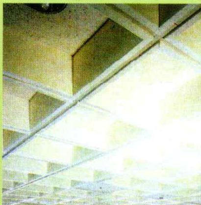
Ceiling suspension bars
